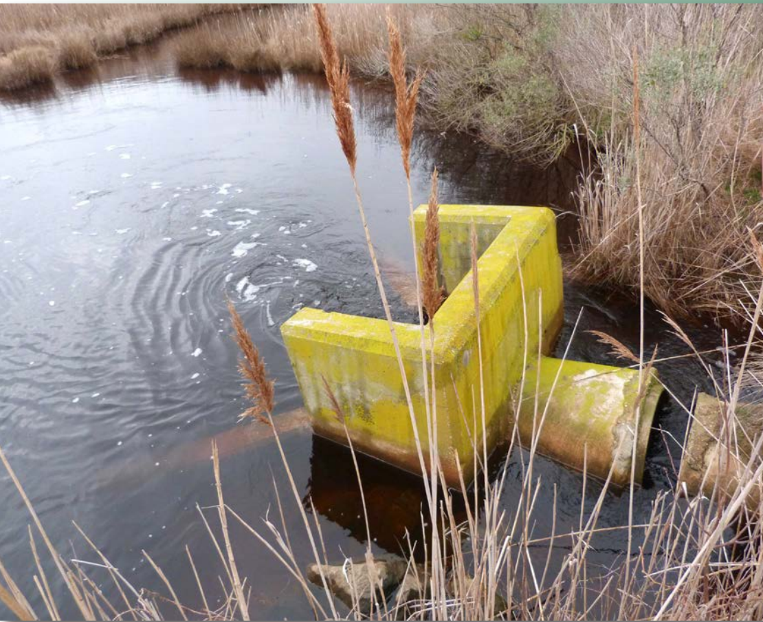
One of the damaged water control structures slated for replacement USFWS
